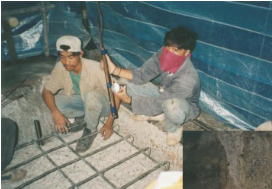
10. 93-12-30: 32 mm \varnothing rods placed in the injection holes with injection and vent tubing attached.
