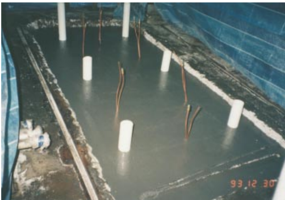
15. After the cement grout had set up, ALPHATEC 800 epoxy grout was mixed and poured overall to approx 60 mm below floor level. This pour also effectively sealed the injection holes, for pressure resistance of up to 300 bar. Injection was carried out on 31 December.
