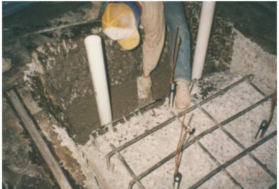
14. ...and the grout poured into the large excavation. The surface of the concrete had earlier been primed with epoxy resins.
